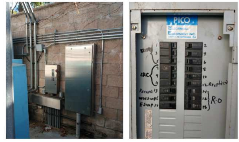
(E) BUS WASH PANEL
